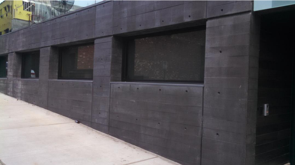
Figure 3. The SCC flowed underneath and between the windows.
