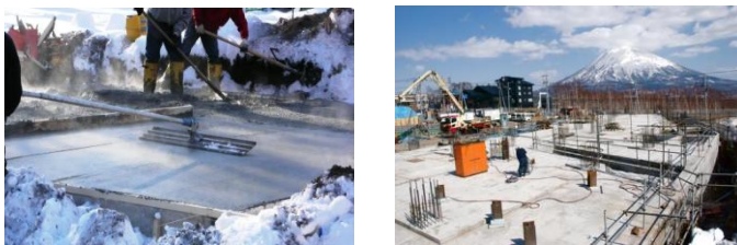
Figure 70. a) placement of concrete in cold weather [1] b) curing of concrete in cold weather [2]
