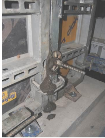
Figure 4. Vibrated concrete – Gap of 7 mm in the vertical joint
