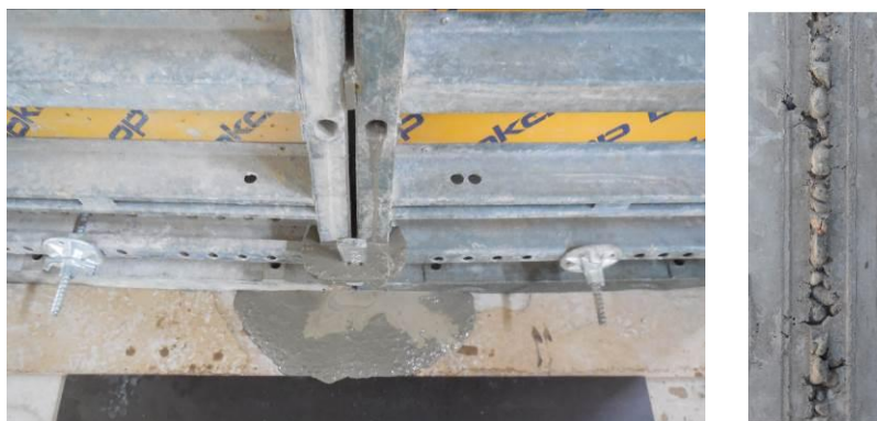
Figure 13. Column 4 – Butt joint with a gap of 9 mm
