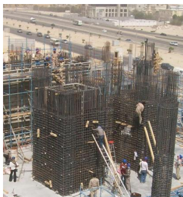
Figure 2. Congested reinforcement in shear walls
