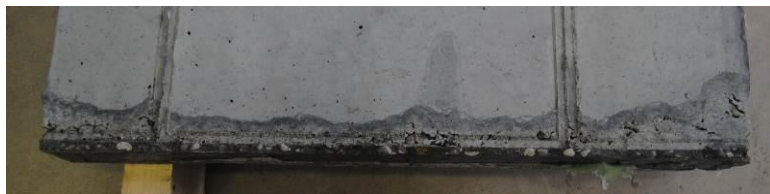
Figure 11. Vibrated concrete – Gap of 9 mm in the horizontal joint
