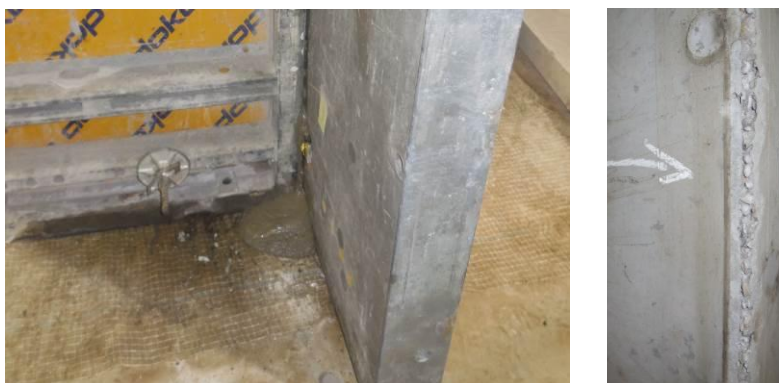
Figure 12. Column 2 – Corner joint with a gap of 9 mm
