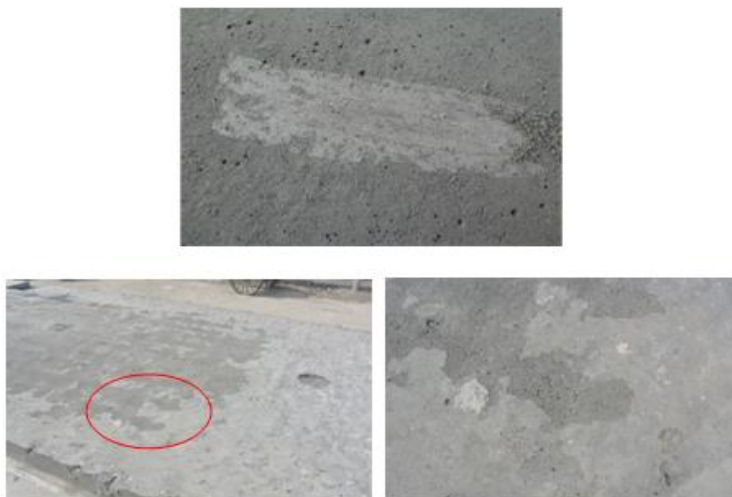
Figure 2. The weak surface of SSFSCC layer after removing prefabricated slab
