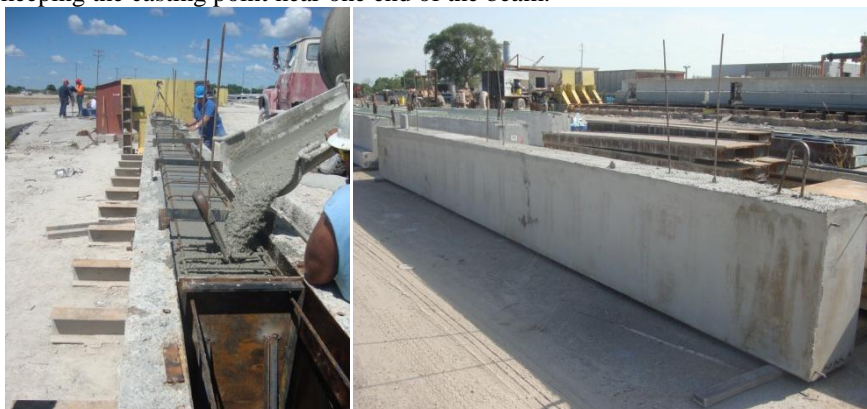
Figure 82. Left: casting of beam 3. Right: beam 5 with the three sets of prestress strands.
