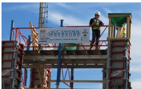
Figure 6. View of “SCC Under Pressure” columns, modified tremie used in concrete placement, and measured-to-predicted lateral pressure
