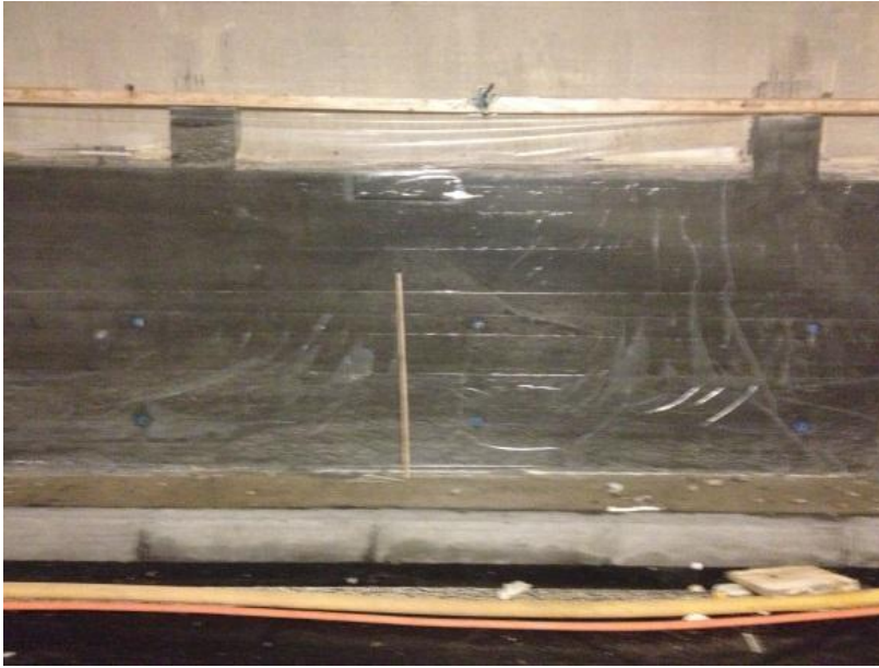
Figure 1: Example of aggregate pile (middle), bleeding marks (left chimney and bottom)
