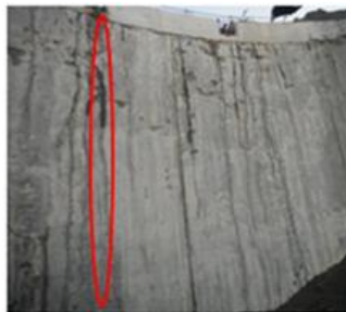
Figure 2. Chimneys of water upwelling or sandy veins
