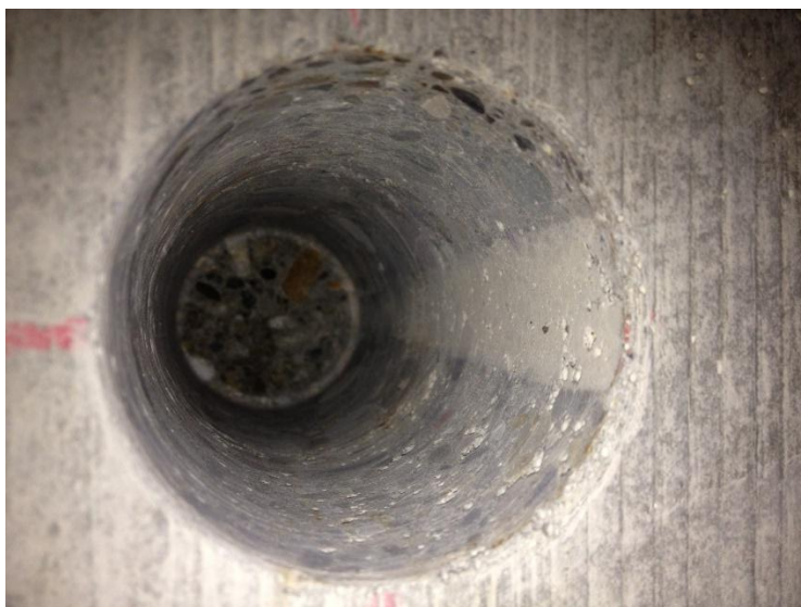
Figure 3: Borehole (image turned 90°), with voids inside the structure
